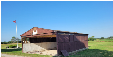
The old pavilion after some salvage for recycling was finished and before it was totally demolished.
