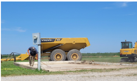
A faithful volunteer cleans the site getting it ready for the concrete pour.
