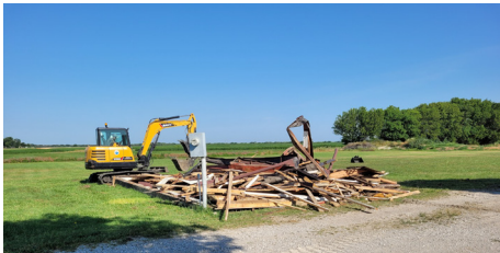
A short time later, the old building is a pile of rubble waiting for clean up.
